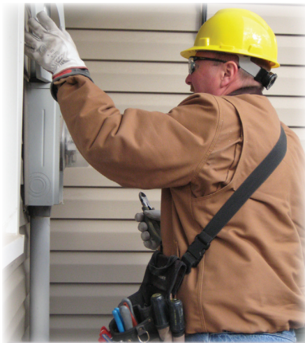
A contracted meter technician replaces an old mechanical meter with a digital "smart meter."
